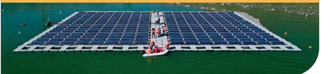
Floating photovoltaic plant in tailings dam
