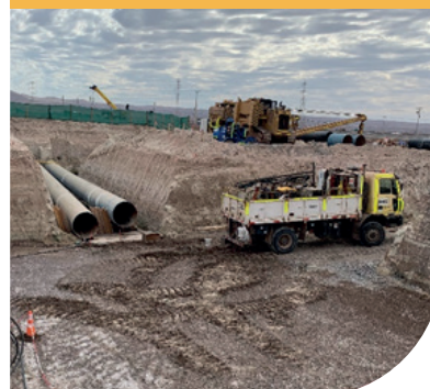
Technical Work Inspection for the Project: "Construction of Collector Pit and Drainage Pool for the Copper Concentrate and Desalinated Water Transportation System (Pipeline)", located at Junction under Route 5. Customer Teck QB2.
