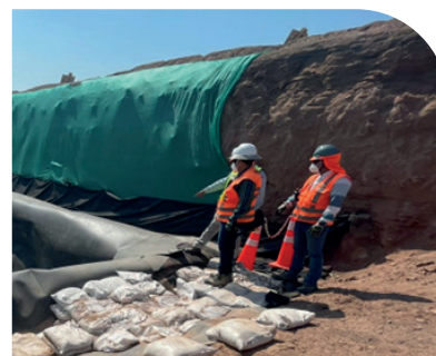
Technical Work Inspection for the Project: "Construction of Drainage Pool and Moat Transport System Collector Copper Concentrate and Desalinated Water (Pipeline)", located at Cruce bajo Ruta 1. Teck QB2 client.
